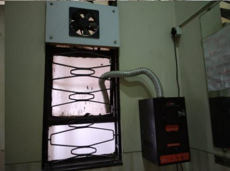
Incinerators for disposal of Sanitary Napkins
